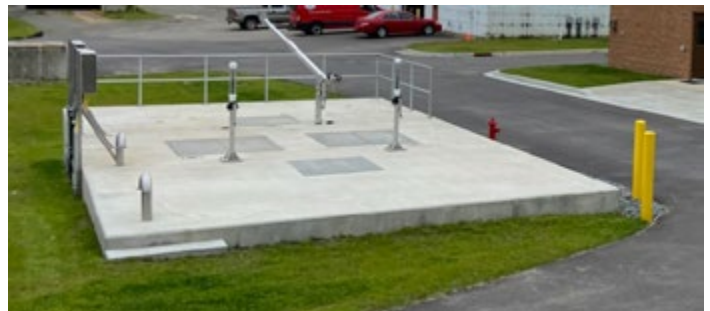
Influent pumping station after upgrade
