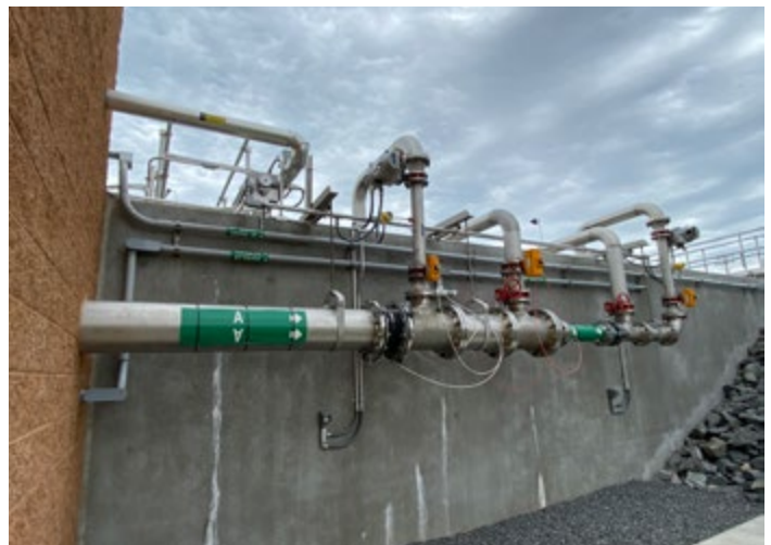
Pneumatic air control valves
