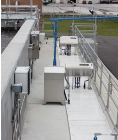
UV disinfection system
