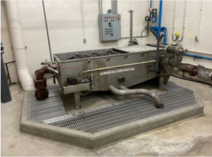
Gravity belt thickener (GBT) curbing and drainage
