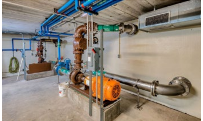
Relocated sludge transfer and loading pump
